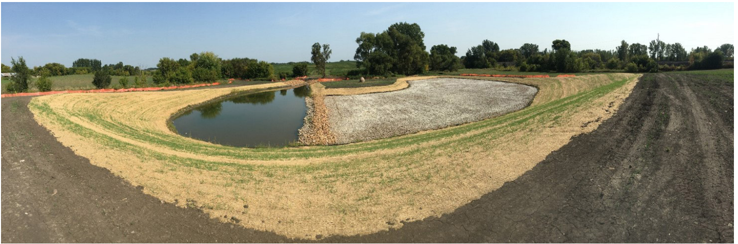
A post-construction view depicts part of the CRWD's Clean Water Fund grant-supported work near Watkins.
