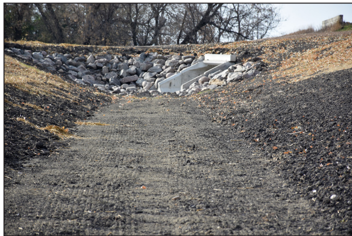
Side-water inlets, top, are part of the BDSWD’s multipurpose drainage management work on Traverse County Ditch 35 supported by a Clean Water Fund grant from BWSR. The project has water storage, water quantity and water quality benefits. Work finished in fall 2022. Above: In Redpath Township, Traverse County Ditch 35 outlets into Twelvemile Creek through a culvert. The ditch, seen here in October 2022, would usually contain water that time of year.
