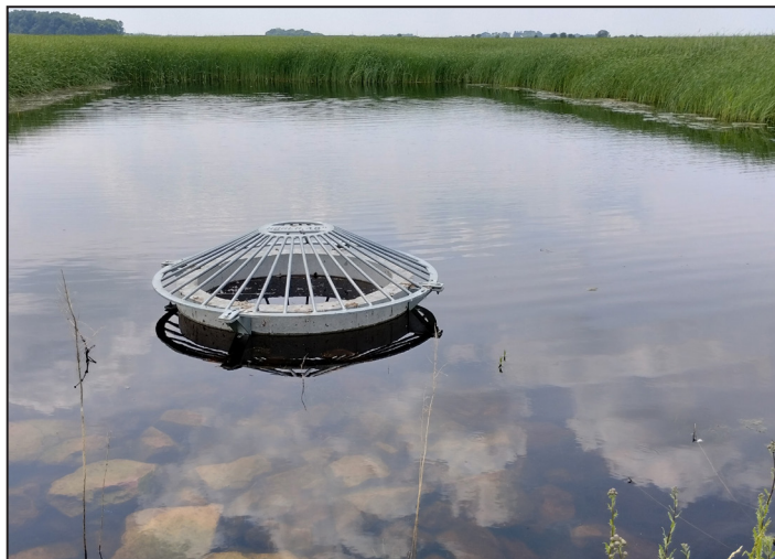
An inlet structure feeds water to a structure containing an internal weir that helps control water levels in the larger of the two restored wetlands. The water control structure connects to County Drainage Ditch 30.
