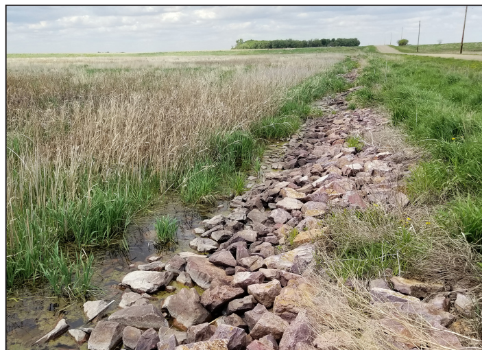
Rock riprap was installed along a township road abutting the restoration site to protect against rodent and wave damage. A stretch of the road was raised and resurfaced during construction. The road's side slopes were flattened to reduce erosion. Photo Credit: BWSR
