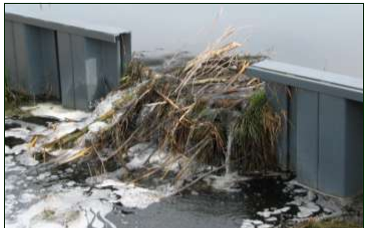
All structures, whether a ditch plug, earthen embankment, or this outlet weir, can require maintenance.
