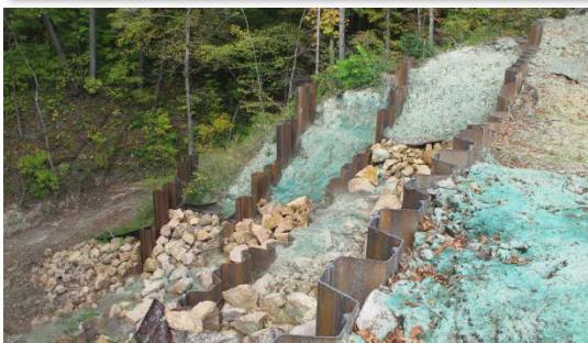
Pictured, top: This July 2014 photo shows significant project damage. Middle: September, after the project had been rebuilt. Bottom: Check dams will help slow water and sediment flow, reducing erosion.
