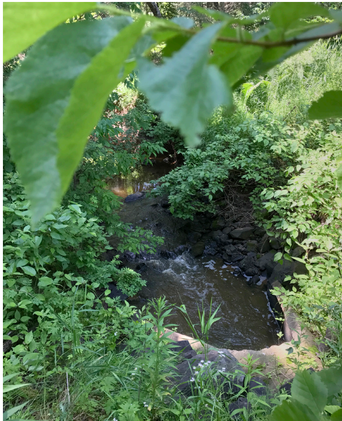
The 1970s structure forced the 20-foot-wide stream through a 4-foot pipe, seen here in 2017. Photo Credit: Ann Wessel, BWSR
