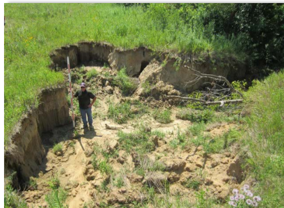
Gully erosion in Dakota County’s Miesville Ravine Park following heavy rains in June 2012.
