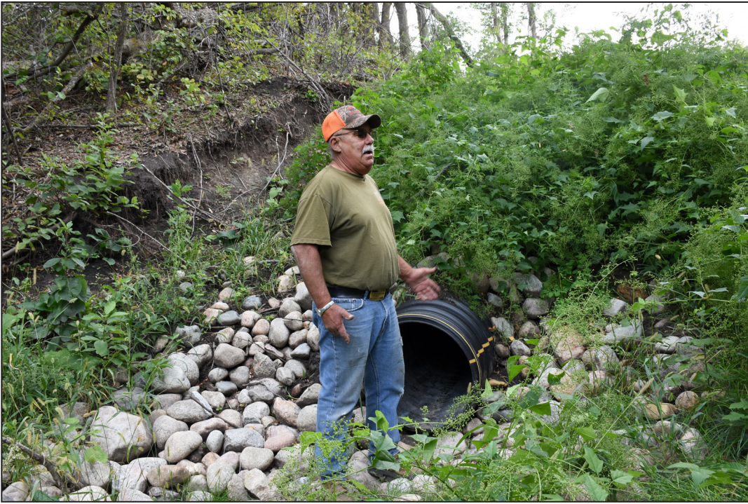
Joe Ste. Marie talked with Red Lake County SWCD staff about the improvements he's seen since a grade stabilization structure was installed at the edge of his Terrebonne Township field. A 30-inch-wide, 130-foot-long pipe now carries water from the field to this point, where it is filtered before reaching a Clearwater River tributary.
