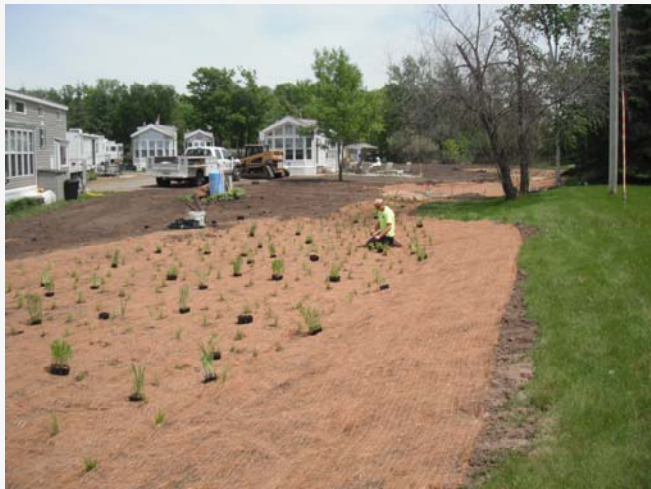
Rain Garden was designed to capture runoff from impervious surfaces at Breakers Resort and Marina on Mille Lacs Lake
