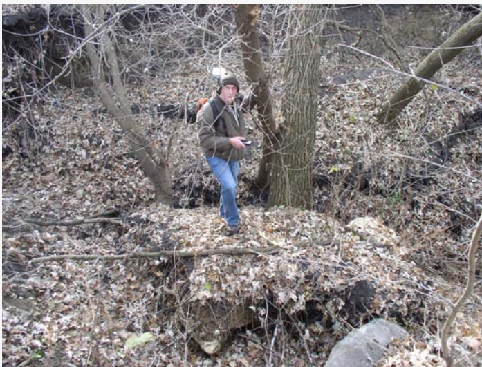
A view down the washout
