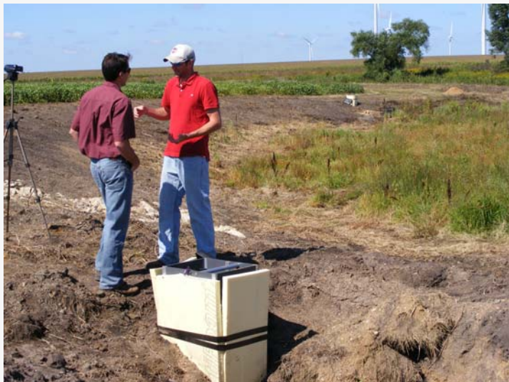
A lowflow bioreactor inlet control structure
