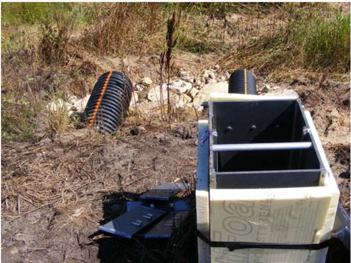
A bioreactor outlet control structure flowing into surge pond and the high flow (bypass) outlet
