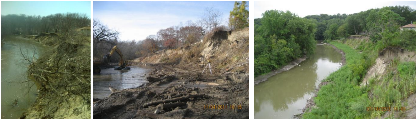
(Picture 1) Bluff 3 had massive erosion prior to project construction. (Picture 2) Crews install natural materials during construction in 2011. (Picture 3) Six months following construction, vegetation has filled in, making the project stronger.
